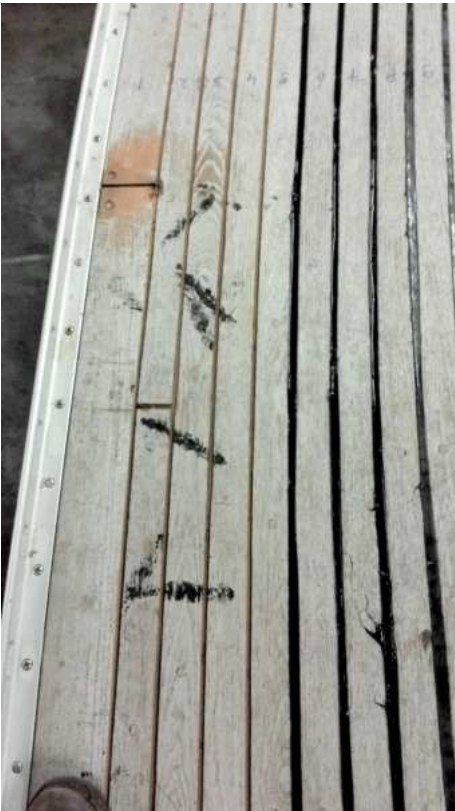
Fig. 17 'Stepped in the caulk' and left traces
